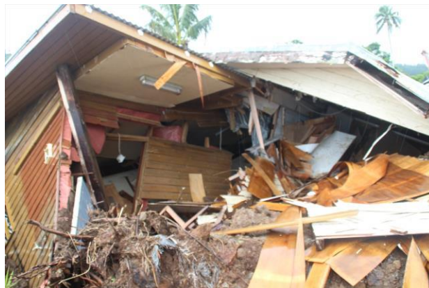
Landslide in Qamea, January 2017
