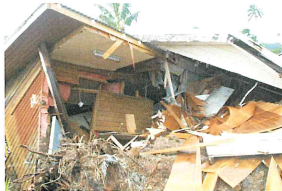
Landslide in Qamea, January 2017
