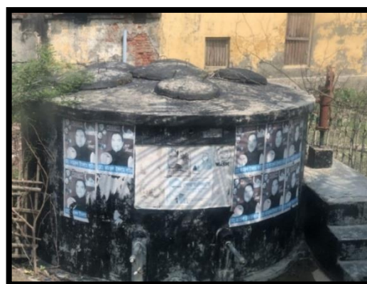
Dysfunctional pond and sand filter
