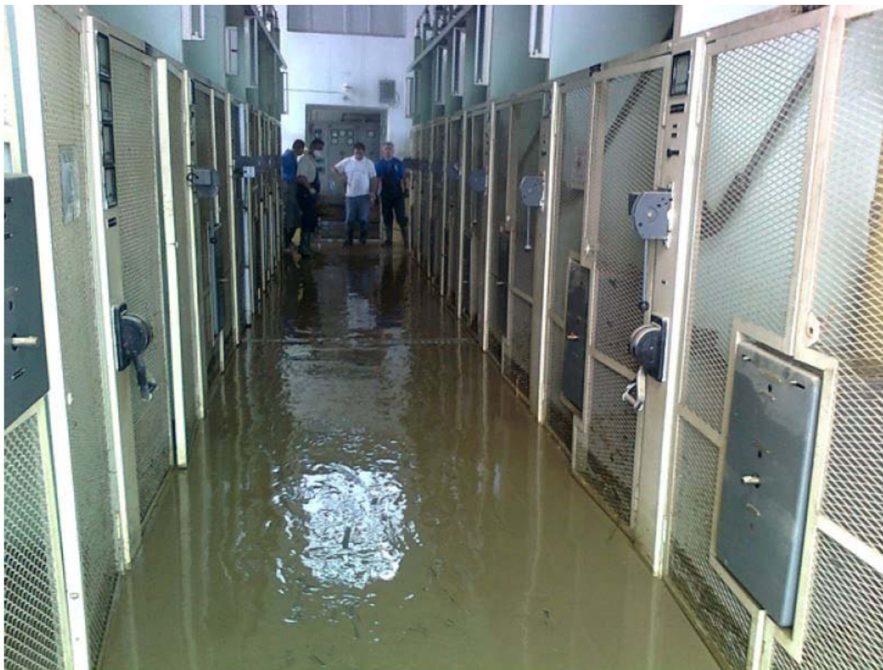
Flooded substation at Orasje. Photo from the Bosnia Floods PDNA report, 2014.
