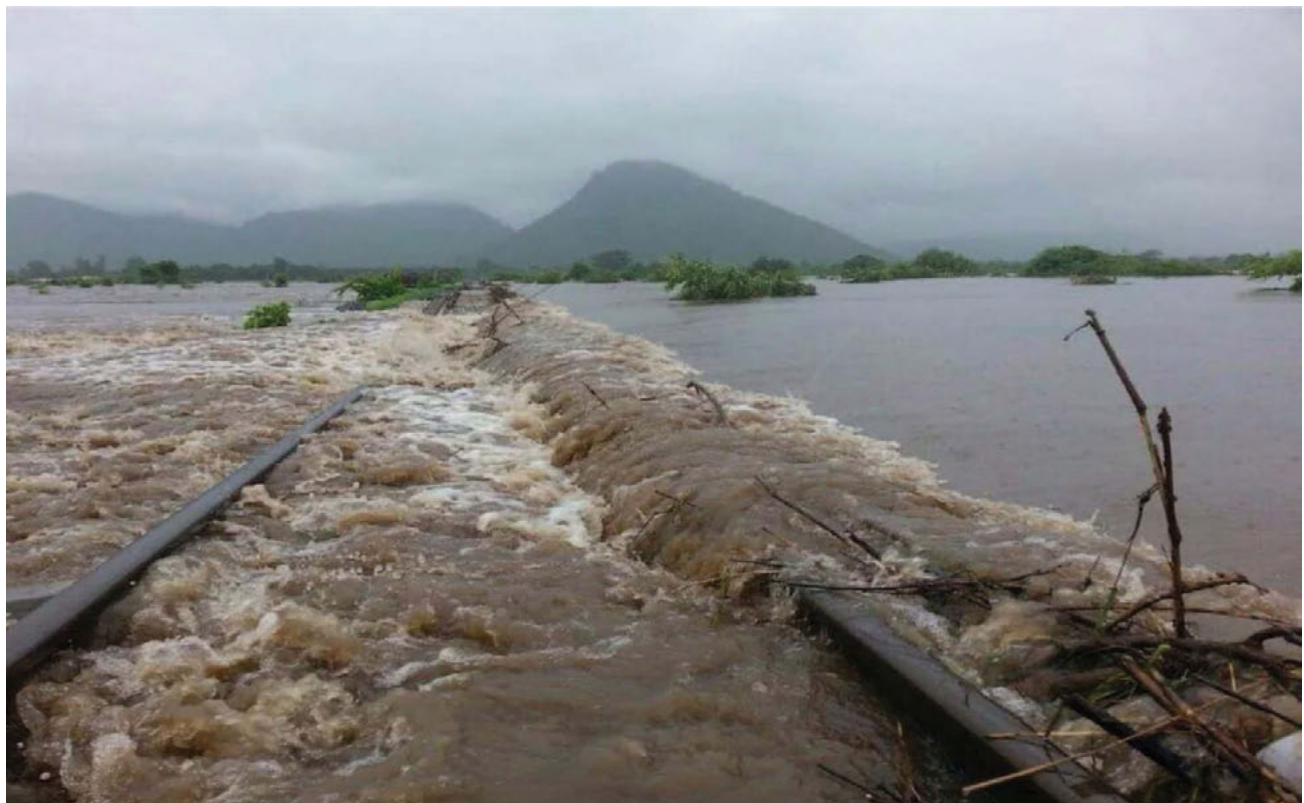
Damages to railways. Photo from the Mozambique Damage Assessment report, 2015.
