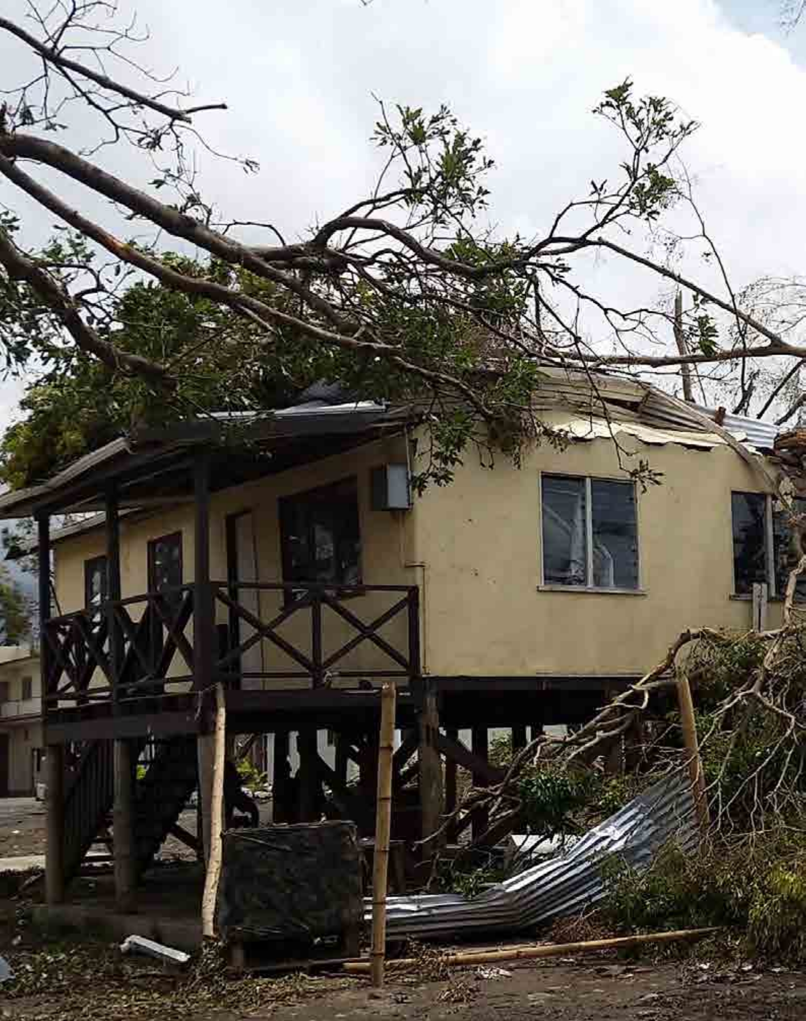
Rakiraki Market (Fiji) - This accommodation centre used to provide rural women market vendors with a safe place to stay overnight when they came to town to sell their produce at the market. A tree brought down by Tropical Cyclone Winston made the structure unsafe and it has had to be demolished.
