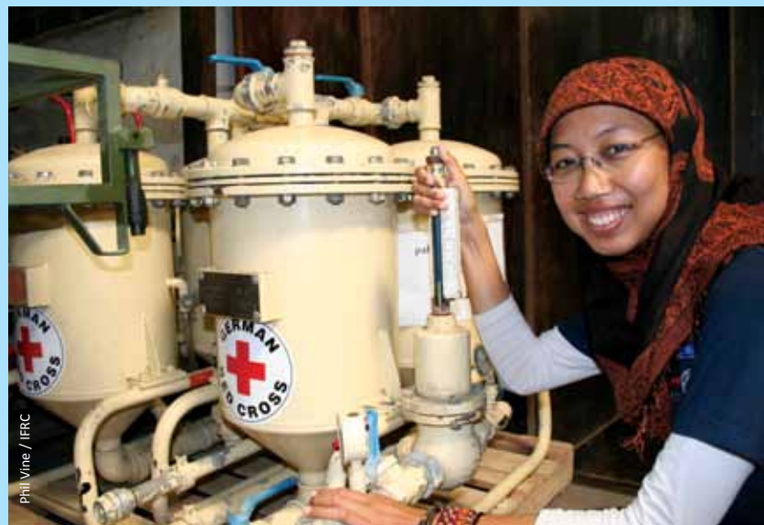
Indonesia Red Cross Water and Sanitation Volunteer inspecting water purifying equipment used in the response to the Yogyakarta earthquake in May 2006.
