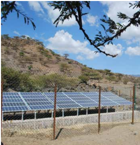
Solar powered multiple and economic uses water for food & household economic security-Ethiopia
