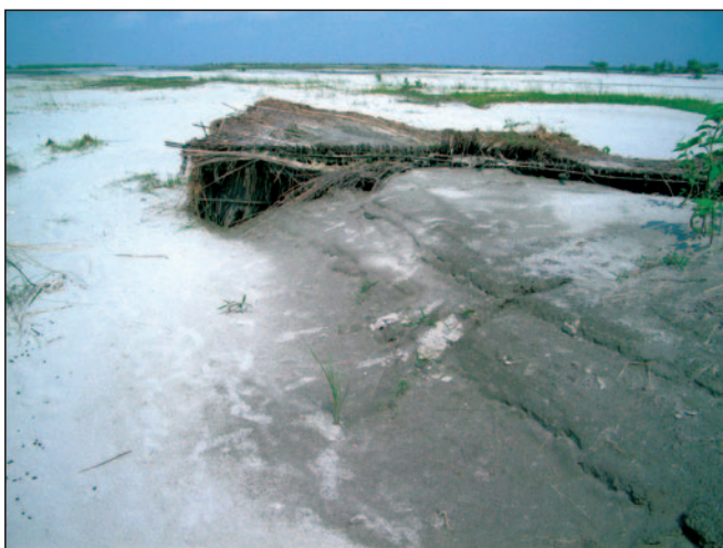
Fig. 21: Destroyed house in Bangladesh 2004 floods
