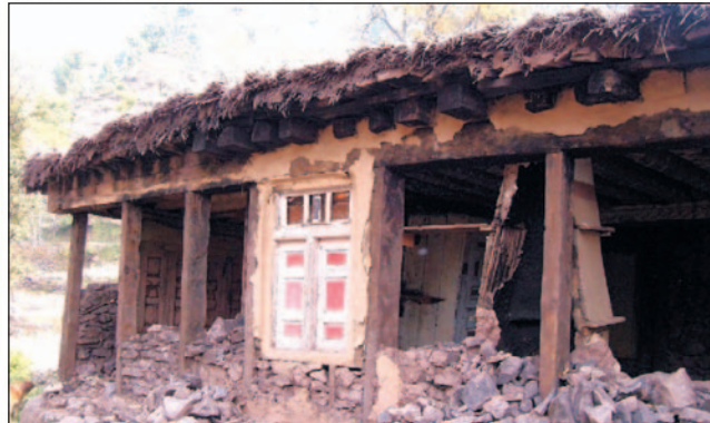
Fig. 29: The house of Waseer in Dachod Faqera, Jhelum valley. The ruins of this house are a good example of what traditional houses at this elevation look like - with stone and mud walls, wooden portals and lintels (still standing and the safest place to be if an earthquake occurs). The wooden ceiling is still intact but the family was unable to survive the falling walls.
