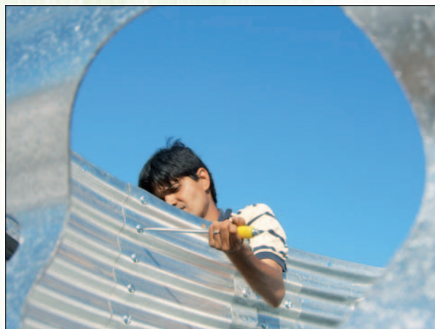
Fig. 35: Mohamed Hilmi, Oxfam Public Health Engineer, helps to construct an Oxfam T11 water tank in 'CTB camp', Kinniya, Trincomalee District, eastern Sri Lanka after the tsunami
