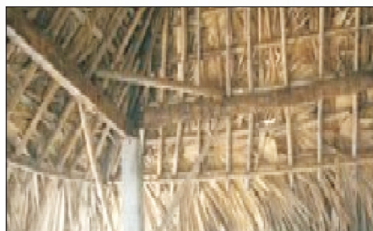
Fig. 28: A traditional house with reinforced cement concrete (RCC) column and corner strengthening
