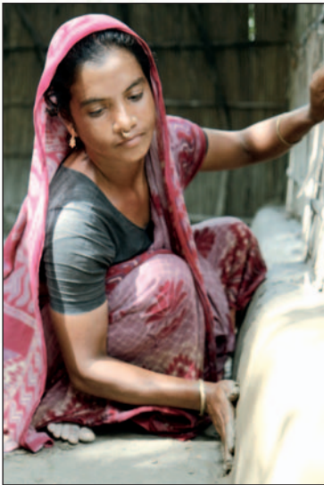
Fig. 23: Dalimon Begum adding more mud to the foundations to raise her homestead which protected her from the floods in 2007
