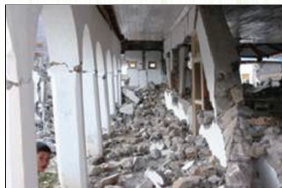
Fig. 9: A devastated hospital in North West Frontier Province, Pakistan after the 2005 earthquake
