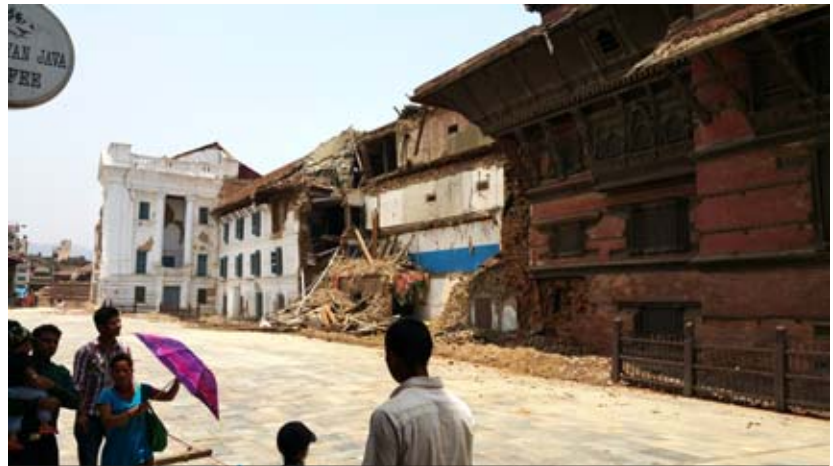
Damage to Hanuman Dhoka Palace Museum due to 2015 Nepal Earthquakes.
